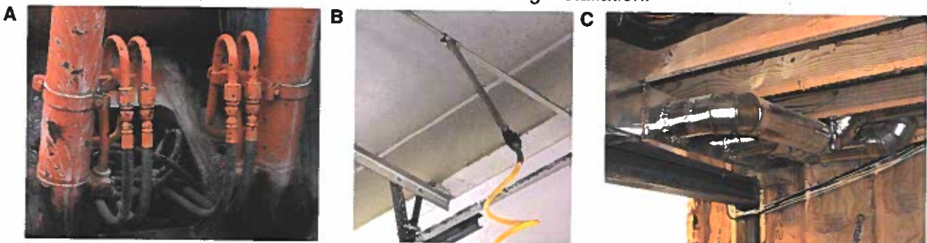
Figure 10-18. Examples of fluid power conductors. A—Flexible hoses allow movement of parts in machines operated by fluid power. B—Rigid piping is used in fixed installations, such as this compressed air system in an auto repair shop. C—Ducting is used to transmit large volumes of air or other fluids at low pressure, as in this forced-air heating installation.
