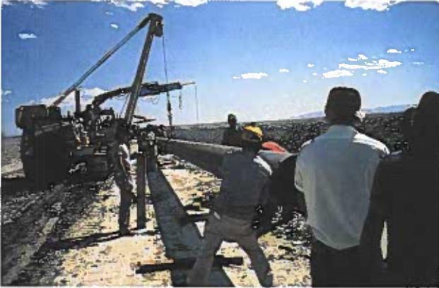
Figure 17-32. It takes many workers and machines to lay a pipeline. (The Coastal Corporation)
