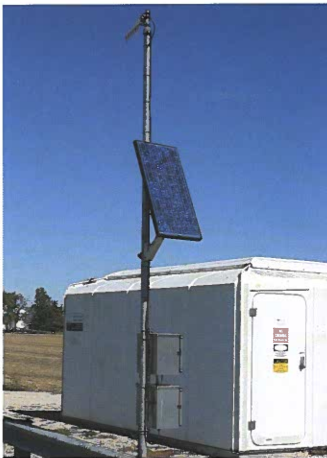
Figure 6-17. Photovoltaic panels are used to provide power in locations where electrical power is not readily available or where a separate power supply is needed that will not be affected by outages of the electrical distribution. This panel provides electricity to power a small radio transmitter that sends data from monitors at a large natural gas storage site. It permits the radio to operate independently and not depend on power from the electrical grid.
