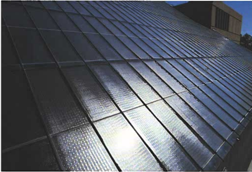
Fig. 7-12. Solar collectors on the roof of this building change light energy into heat energy, supplying most of the hot water needs of the owner.
