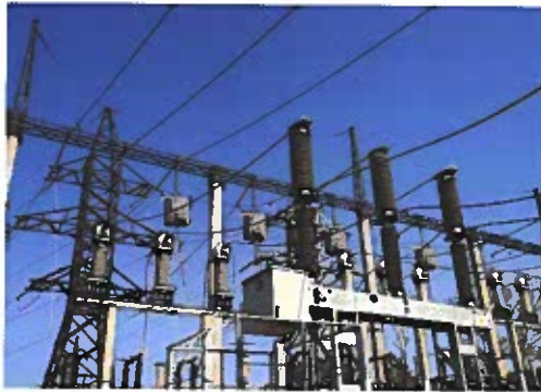
Figure 11-10. Distribution substations step down the voltage.
