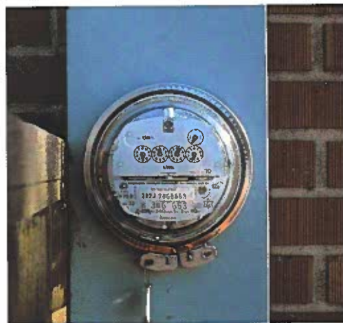
Figure 12-25. A utility meter measures the amount of electricity used in kilowatt-hours (kWh).
