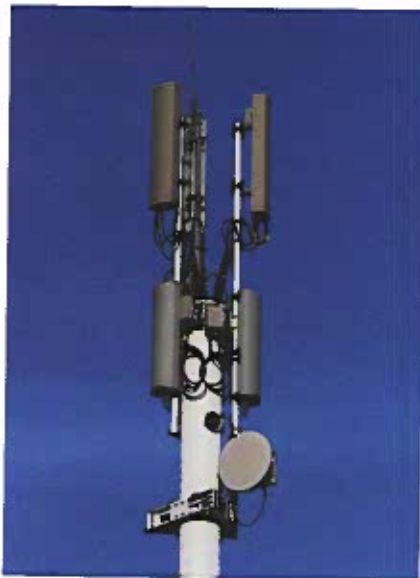
Figure 13-11. A transmission tower with cellular antennas receives and transmits radio signals on the cellular frequencies assigned to its cell.
