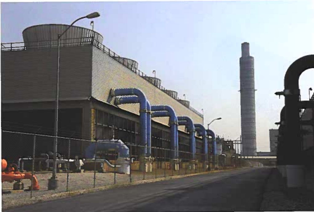
Figure 16-16. Many coal-burning power plants have begun using scrubber technology to minimize air pollution.
