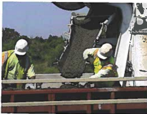
Figure 17-3. Traditional construction workers work for companies that build structures of all kinds. These concrete specialists are pouring the concrete for a new bridge.
